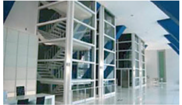
Thermal insulation glass walls applied to refuge stairs
